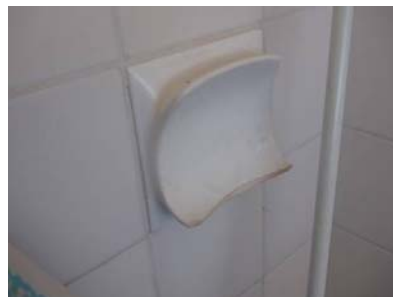
This broken soap dish in the shower could cause injury and needs to be replaced.
